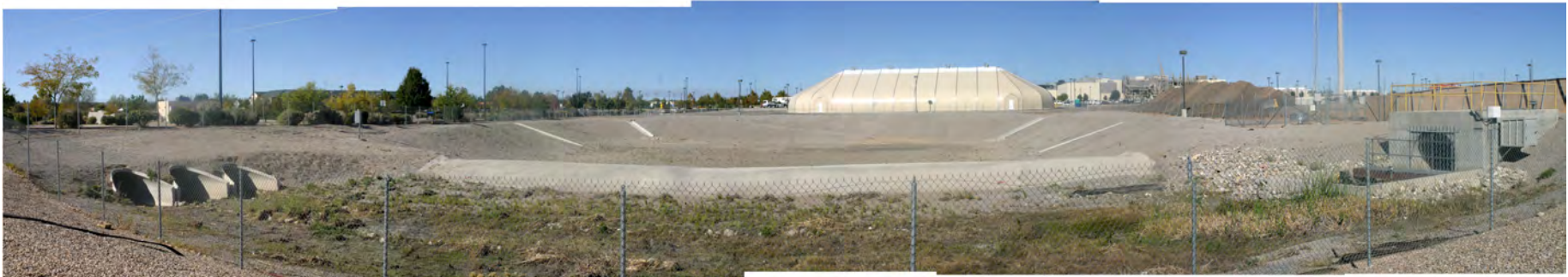
Figure 3 Stormwater detention basin on the Intel campus in Rio Rancho, NM
