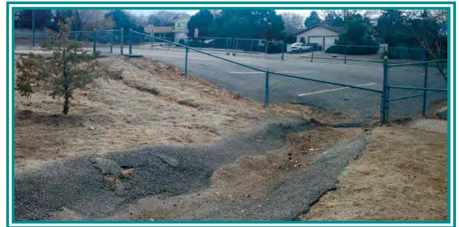
Erosion and Tree Death Due to Poor Slope Management
