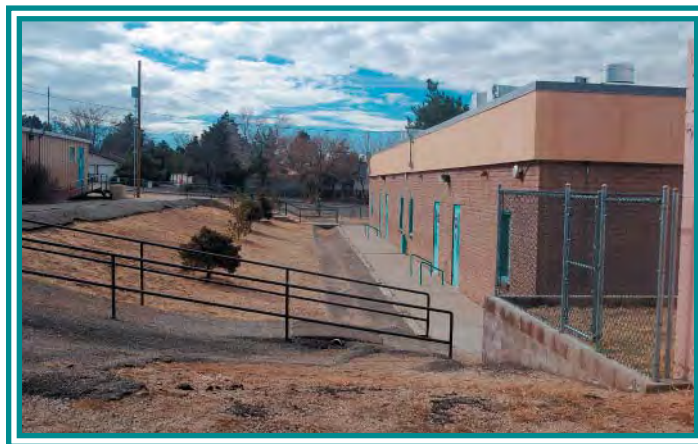
An Asphalt Ditch Channels Water From East Campus to the Parking Lot and Street
