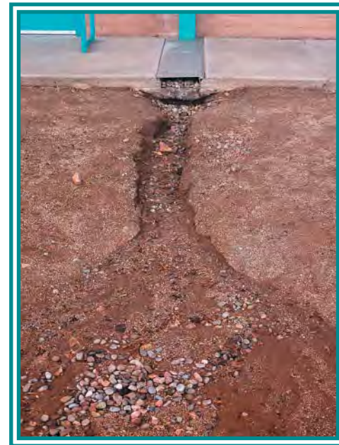
Eroded Drainage Channel
