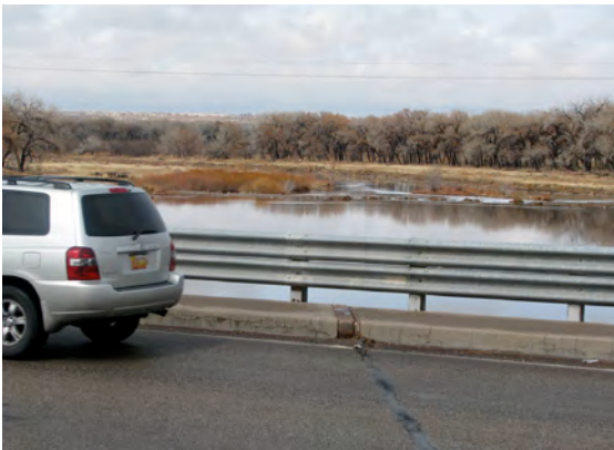
Existing bridge conditions are dangerous and obscure the basin bottom
